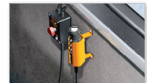
Pit connection box with E-Stop
